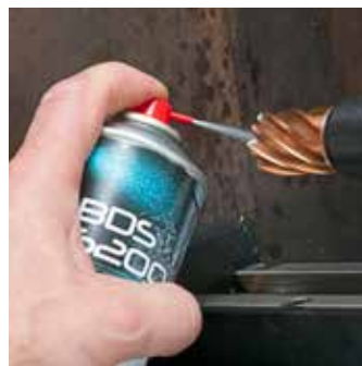
Step 1: Prior to drilling, spray the high-performance lubrication spray directly into the drill.
